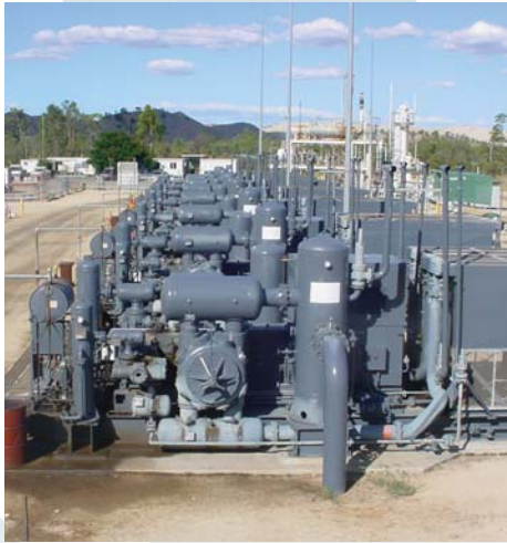
Meridian SeamGas - Hillview compressor station
